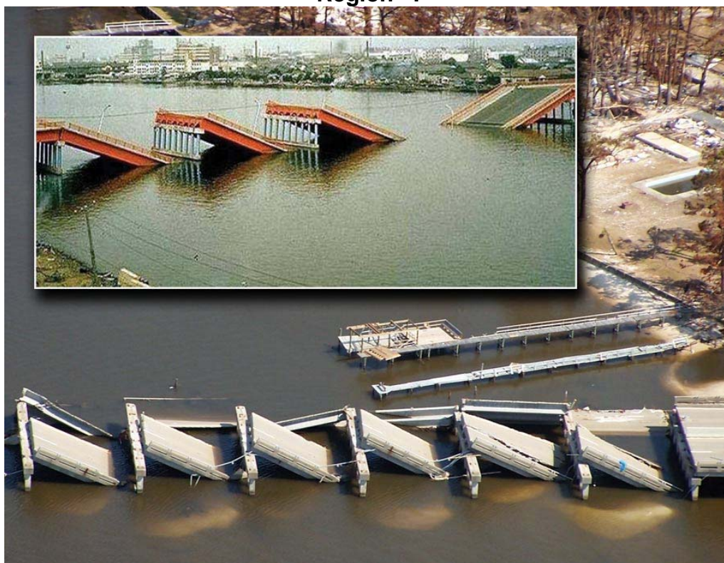
Figure 7: Impact of Hurricane Katrina to Bridges along the Gulf Coast Region 17 :
